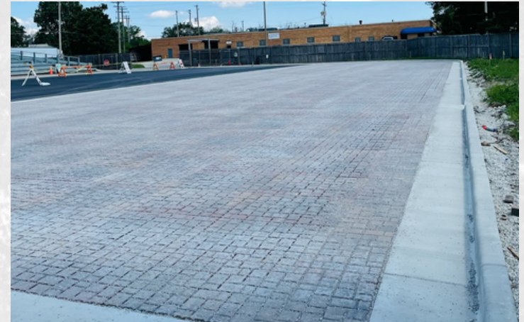
Permeable brick pavers along with curb and gutters were constructed at the recycling center as part of a green infrastructure project with funding from MMSD.
